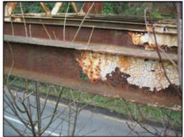
Deck beams, note corrosion of both flanges and web
